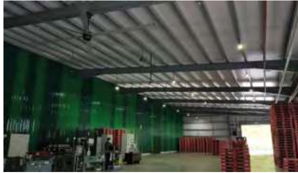
HVLS fan installed at pallet inspection area
